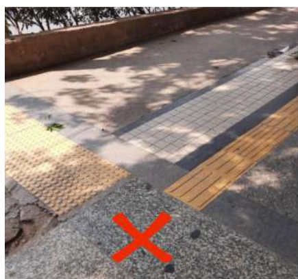
Inaccessible & Improper way of laying of TGS
