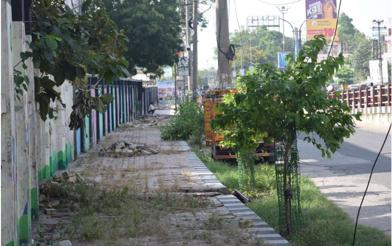
Image 5.7: An ill maintained footpath near Shankar Vilas Railway Over Bridge
