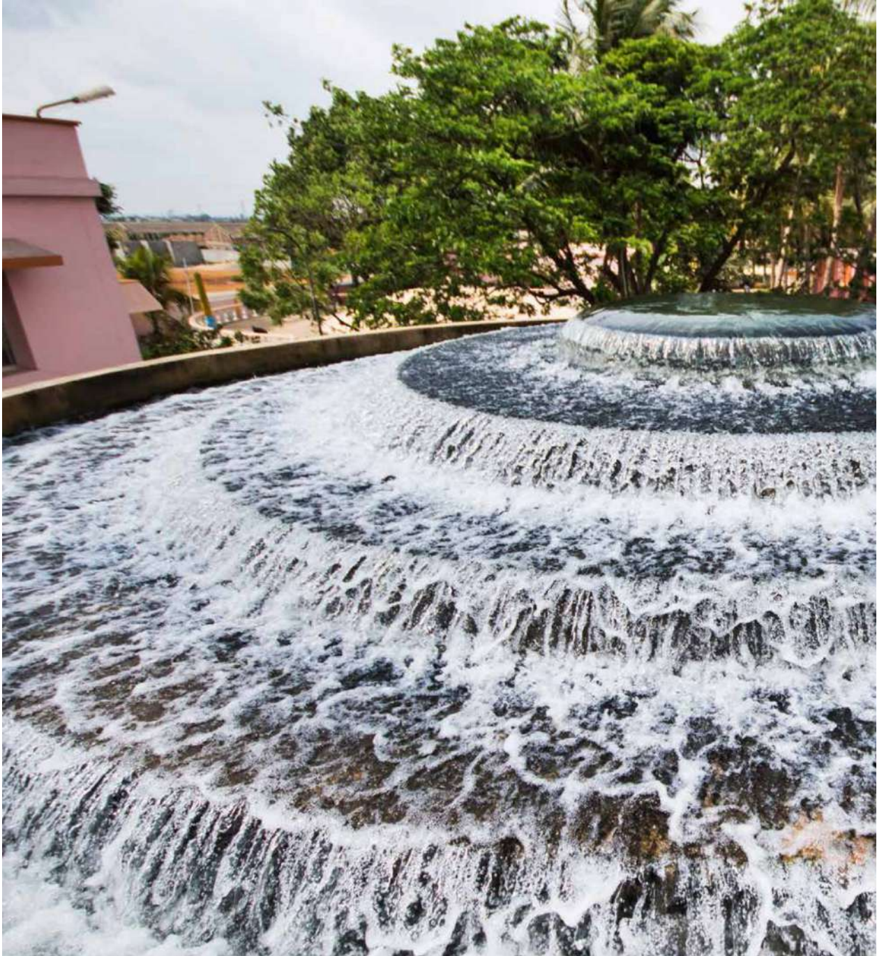
Image 4.10: View of water being treated in Takkellapadu Water Filtration Plant
