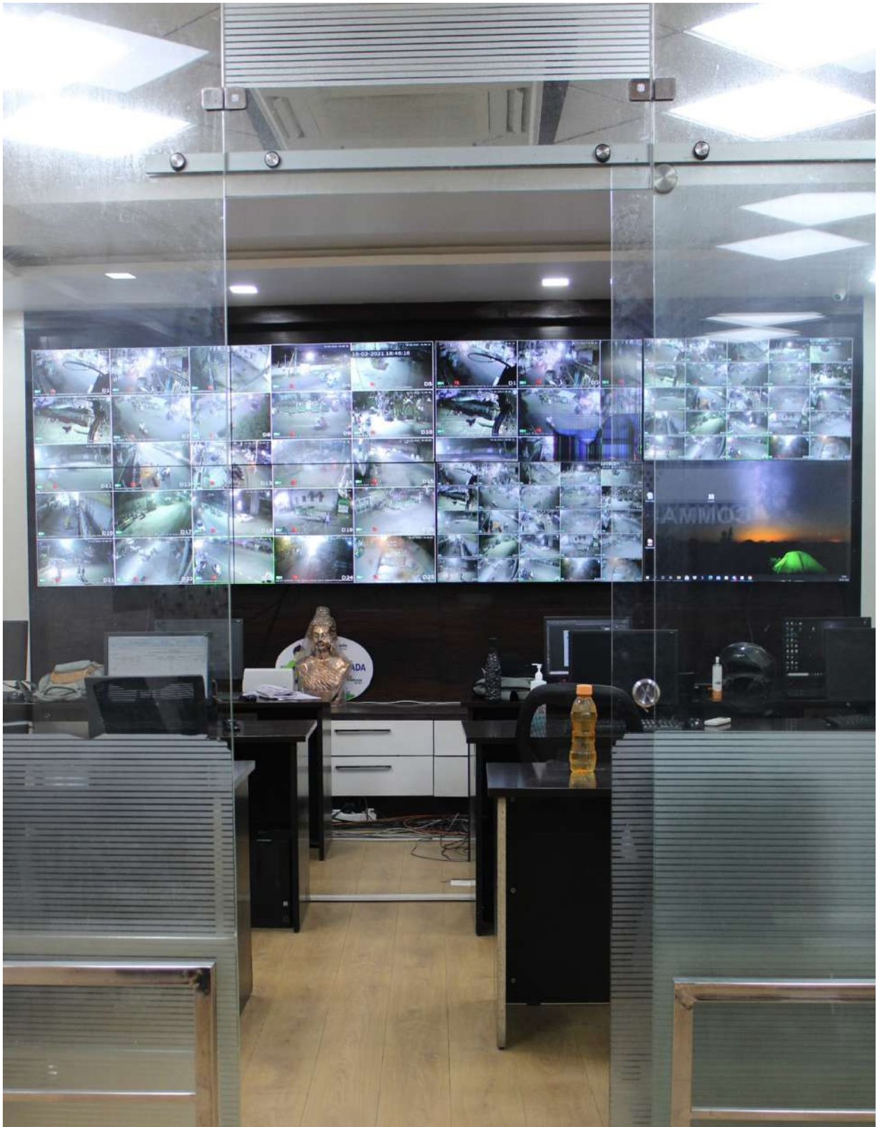
Image 4.31: View of VMC Command Control and Communication Centre (Non-Smart City)
