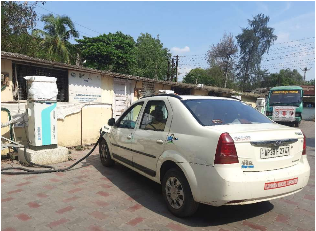
Image 4.29: EV charging stations and electric cars on lease at VMC Office
