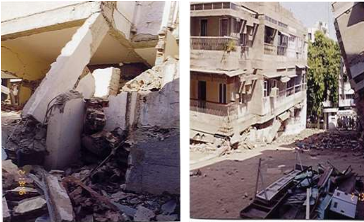
Failure and collapse pattern
