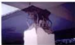
Failure between Beam-column joint
