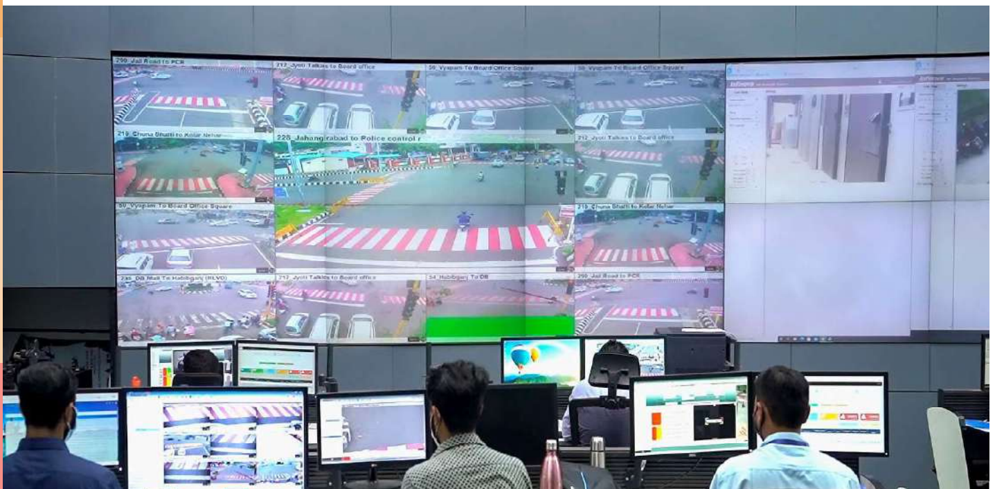
Integrated Command and Control Centre in BSCDCL Office, Govindpura
