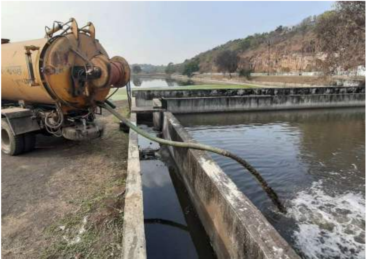
Image 4.10: Vacuum tanker emptying faecal sludge collected from onsite sanitation facilities at Kotra STP
