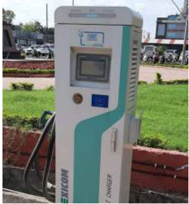
Image 4.14: Pilot electric vehicle charging points in ISBT, Habibganj
