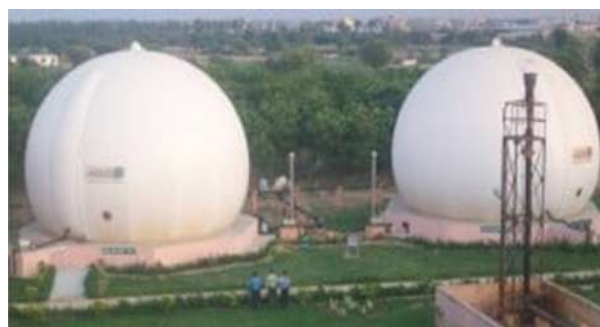
Image 4.16: Gas collection chambers at Delawas STP Source: https://civildigital.com
