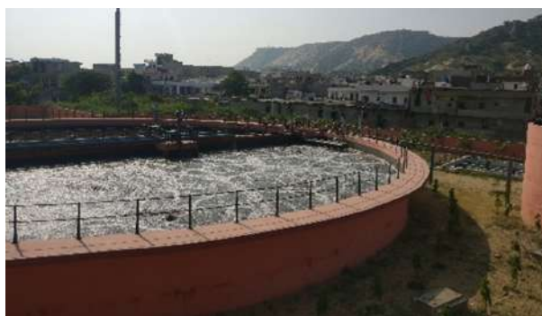
Image 4.13: 8 MLD STP at Brahmpuri
