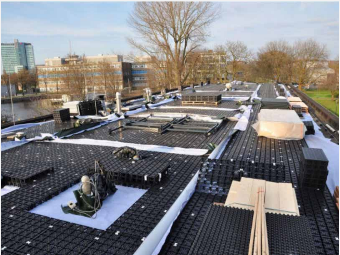
FIGURE 3.58 Project SmartRoof 2.0 rooftops
